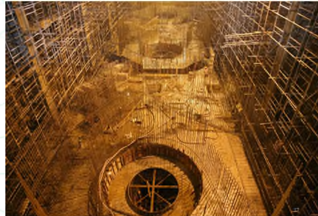
Underground Power House
